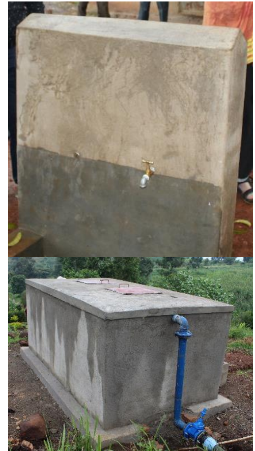
Photo: Some of the new infrastructure included a Break Pressure Tank and Public Stand Posts
