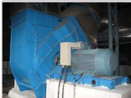
MVR Fan-Heart of the system
