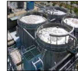
Moving Bed Bio Reactor (MBBR)
