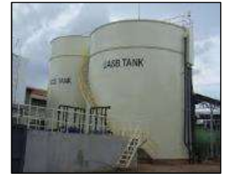
Upflow Anaerobic sludge blanket reactor (UASB)
