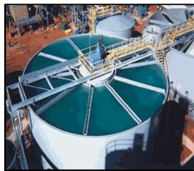
High rate solid contact clarifiers
