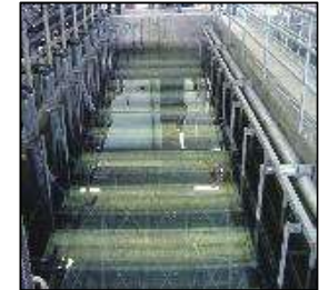
Membrane Bio reactor (MBR)
