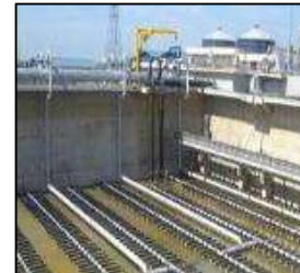
Sequential Batch Reactor (SBR)
