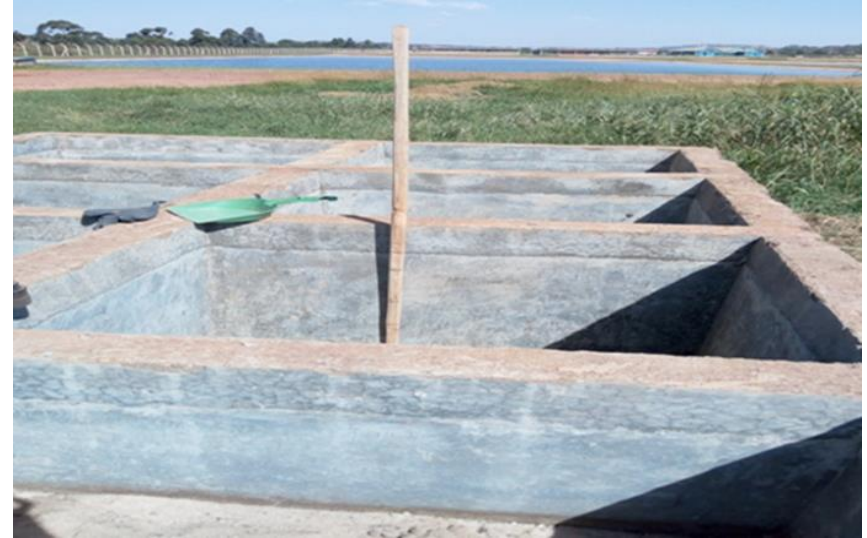
Sludge drying beds constructed for research
