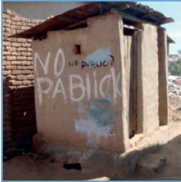
▲ Latrine - before situation
