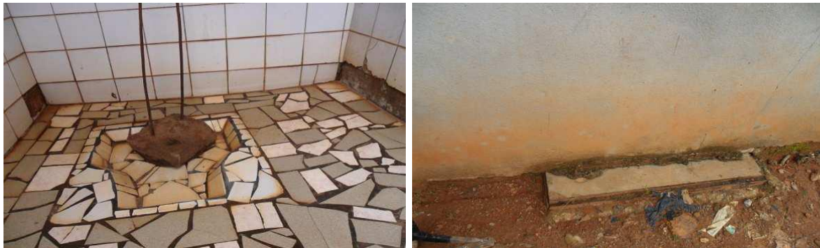
Figure 7 : Household latrines used as "containment". The network of Mendong (left) and house constructed above the network (right) (picture from Mbée, 2011)
